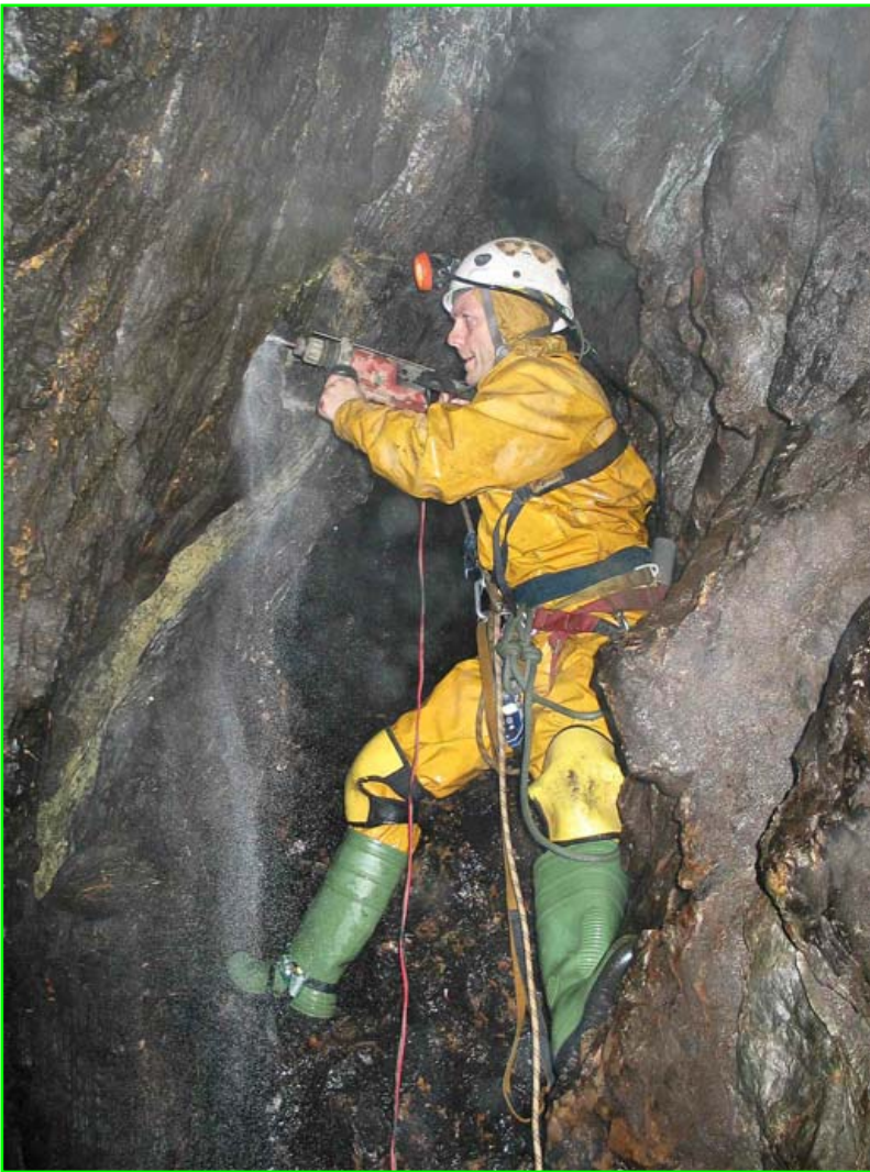
Mark Lonnen Drilling Hole for Eco-anchor in Uamh nan Claig-ionn, Argyll. July 2007.
