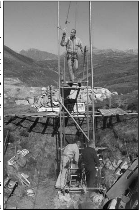
Mark fettling the headgear while Norman adjusts the ‘Fluxcavator Mk 5’ cycle winch.
